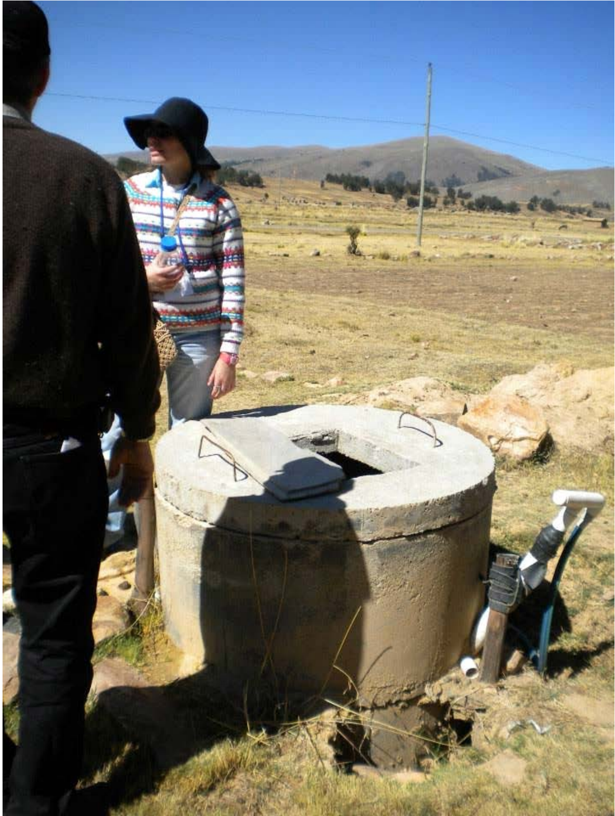
The hole next to the well is a safety hazard as well as a possible means of contamination.
