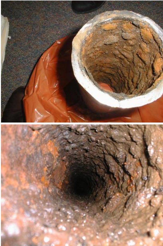
FIGURE 3. RN PIPING TUBERCLES DUE TO RAW WATER SCALING INCREASE PIPE ROUGHNESS AND REDUCE PIPE DIAMETER
