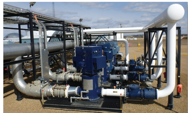
Figure 1 - Crude oil booster pump system
