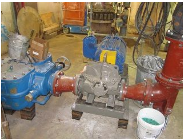
Screen Wash Pumps
