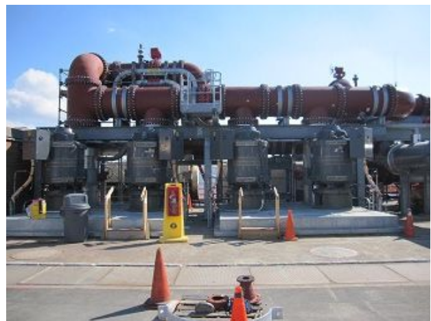
Pump Motors and Discharge Pipe
