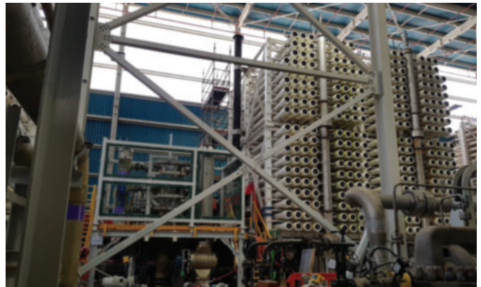
Figure 1: Image of one of the nine Reverse Osmosis (RO) racks as the chimney was being installed.
